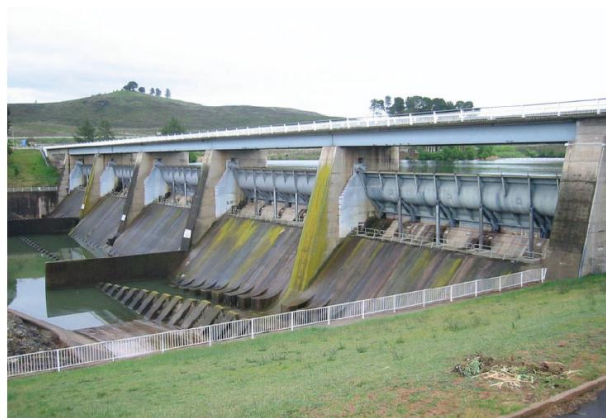
The Scrivenner Dam (an embankment dam) in Canberra which holds back the waters of Lake Burley Griffin. It has been designed to withstand a one in 5000 year flood.
